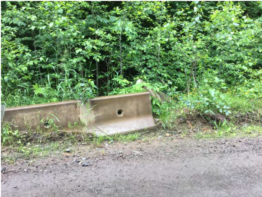
Left upstream approach concrete no post barriers should be realigned
