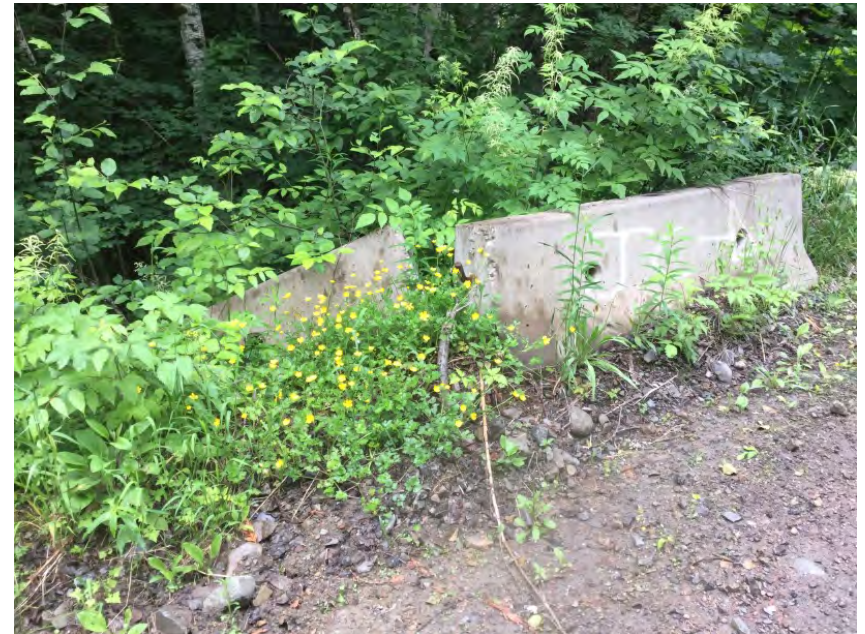
Left downstream concrete no post barriers should be realigned
