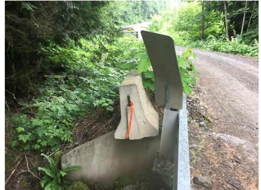
Right downstream approach concrete no pos barriers could be realigned
