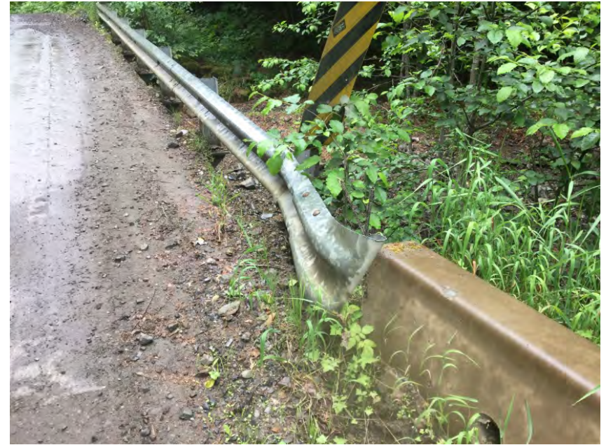
Damage to right downstream guardrail - still functional
